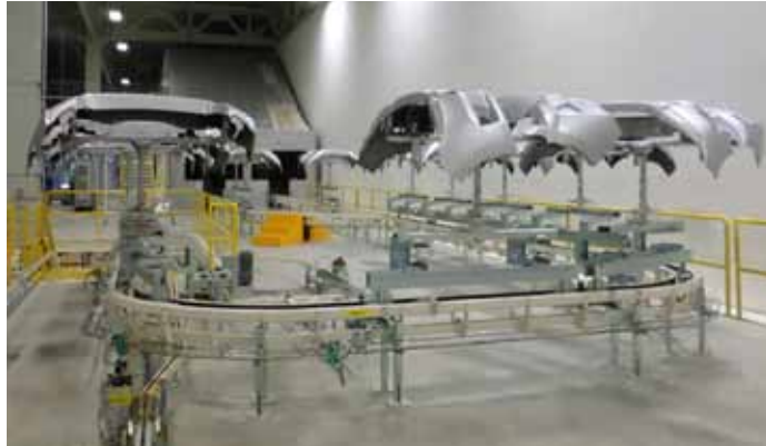
Caldan P&F100, power & free floor conveyor - operating in Mexico - surface treatment of auto bumpers ←
