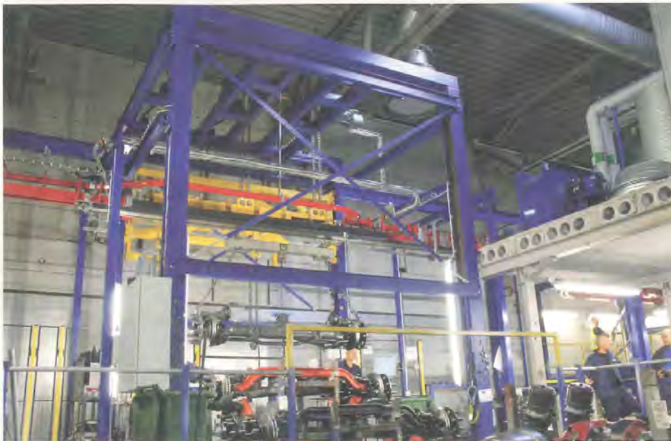
Loading station with hoist to take the axles from the floor to the Power+Free conveyor
