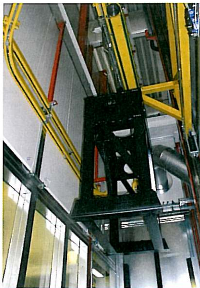
Due to the limited space available, the drying oven at the company Rosenbauer is located on level 6, above the coating booths. The racks are transported there by a lift. The picture shows the conveyor mechanism in the lift.
